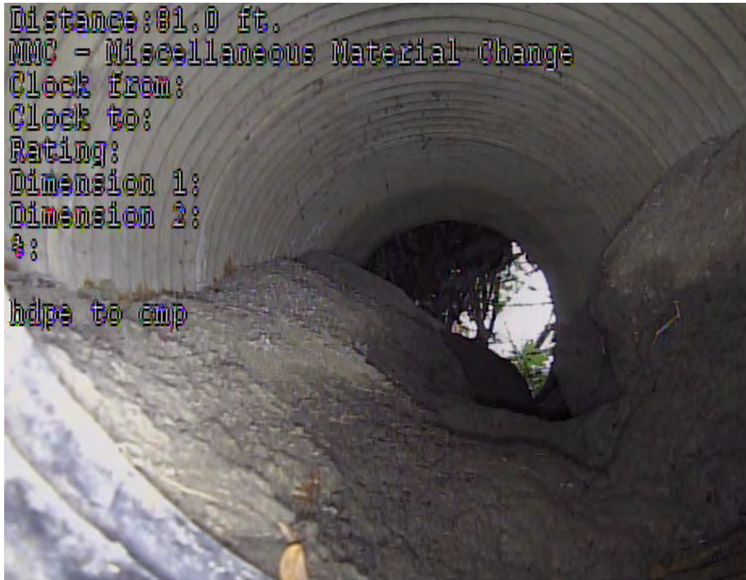
Figure 5-27: Corroded CMP and Outfall Blockage (4 th Street Outfall)
