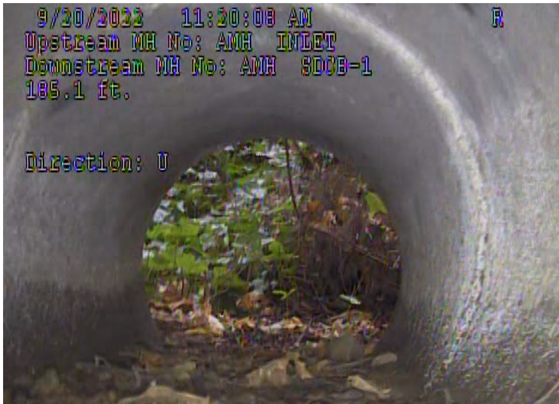
Figure 5-30: Overgrowth and Sediment Accumulation at Upstream end of 6 th Street (24-inch RCP)
