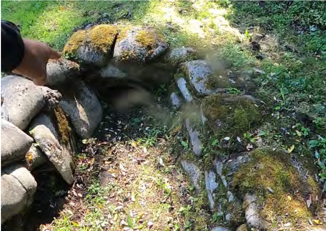
Figure 5-26: 4 th Street Outfall Daylight Section Sediment Buildup
