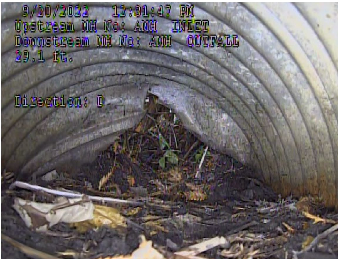
Figure 5-33: Failed 18-inch CMP Culvert at Willow Way (Downstream End)
