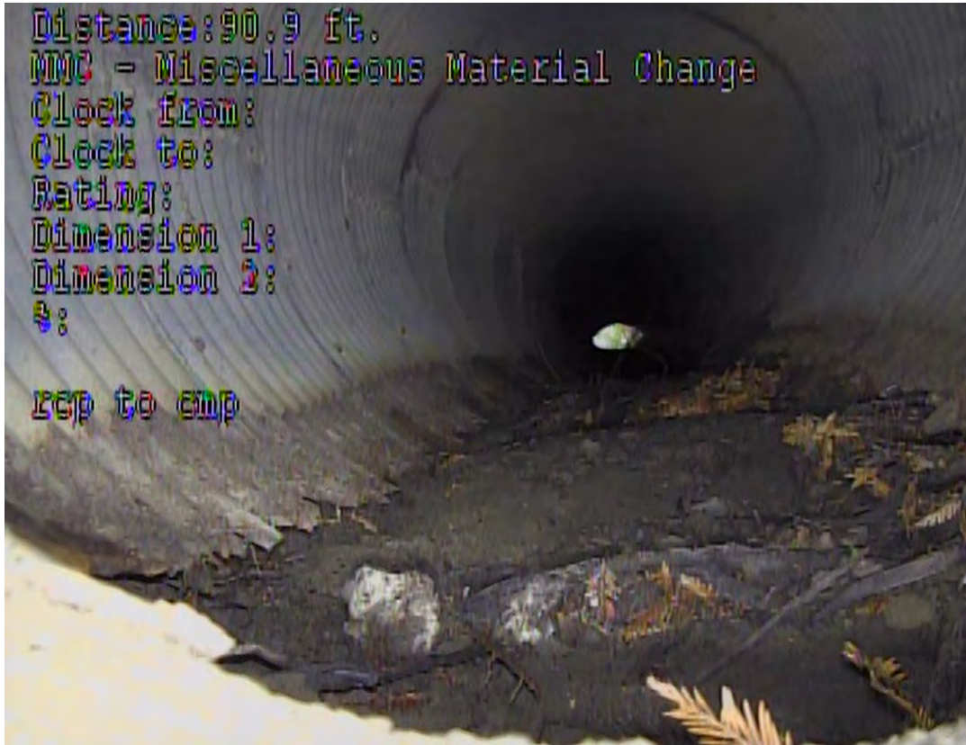
Figure 5-31: Corroded CMP Bottom at Transition from RCP to CMP (6 th Street Outfall)
