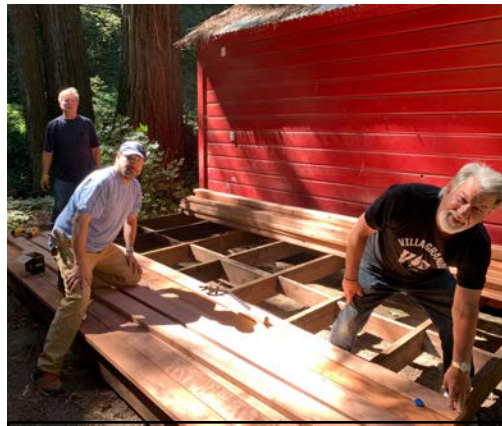
Villa Grande volunteers Rich Holmer, Ruben Garcia and Jon Box working on the platform decking.
